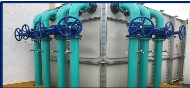
Industrial Water Treatment
